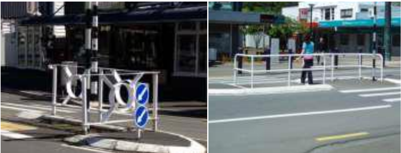
Figure 4.112: Sharp edges on pedestrian fencing
