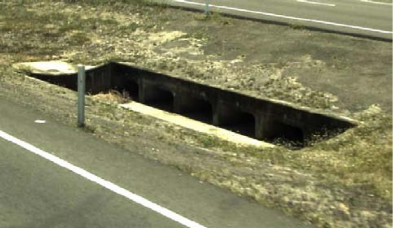
Figure 4.119: Culvert drop in centre median
