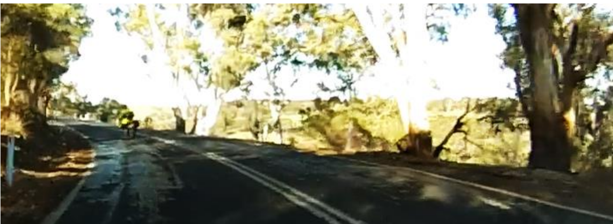
Figure 4.49: Aggregate stripping on curve
