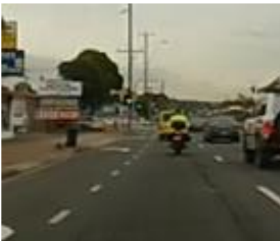
Longitudinal crack on intersection approach
