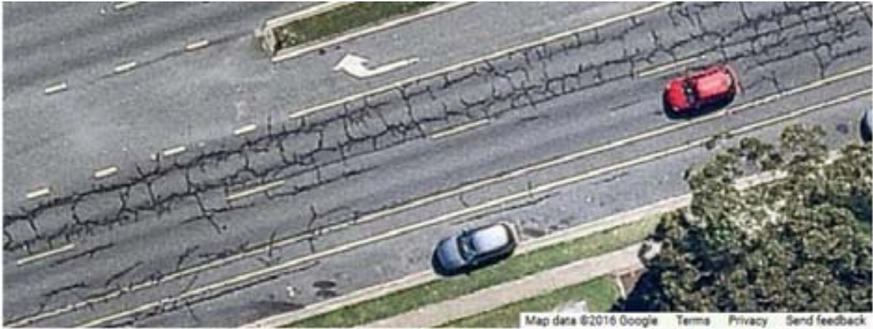
Figure 4.50: Excessive amount of crack sealant
