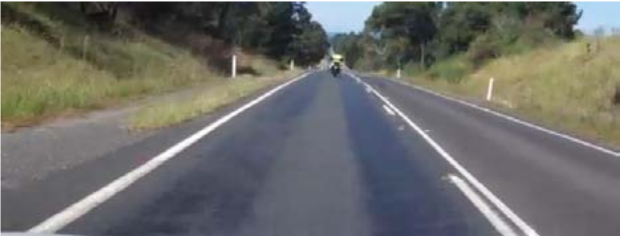
Figure 4.48: Bitumen flushing in the wheel paths
