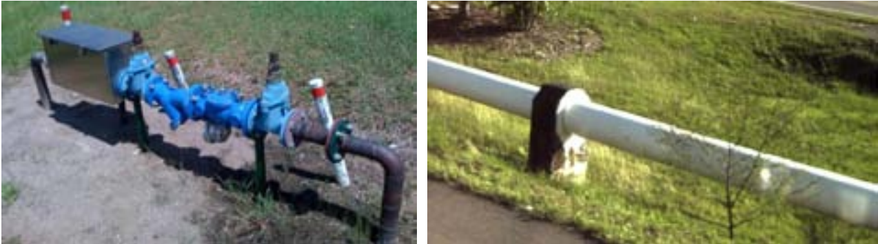
Figure 4.115: Above ground water and gas pipes and meters
