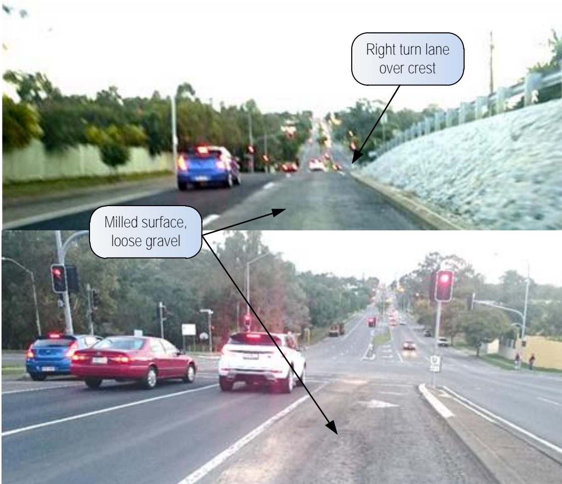
Figure 4.59: Road works, milled surface with gravel spill from asphalt works in through lane and right turn lane
