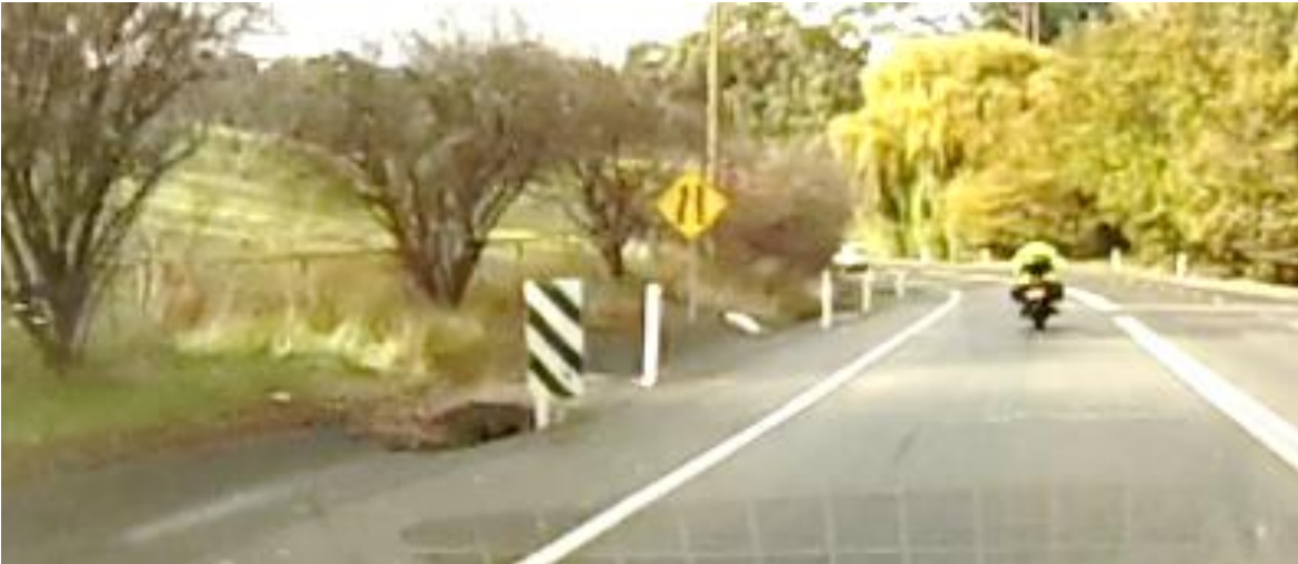
Figure 4.29: Hazard sign on perpendicular culvert
