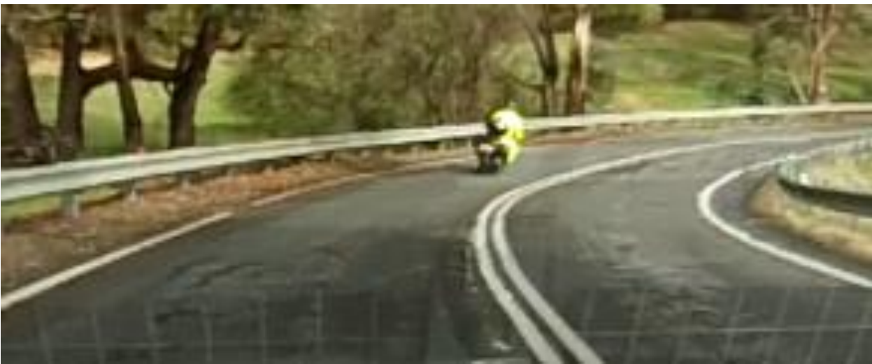
Figure 4.65: Deteriorated pavement on curve (ravelling and stripping)
