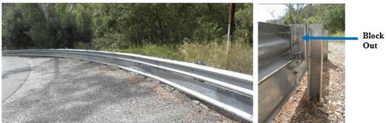
Figure 2.6: Motorcycle protection steel rail
